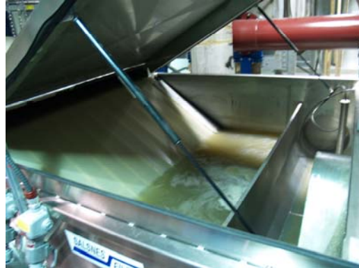
Primary screening system in Iqaluit waste water treatment plant
